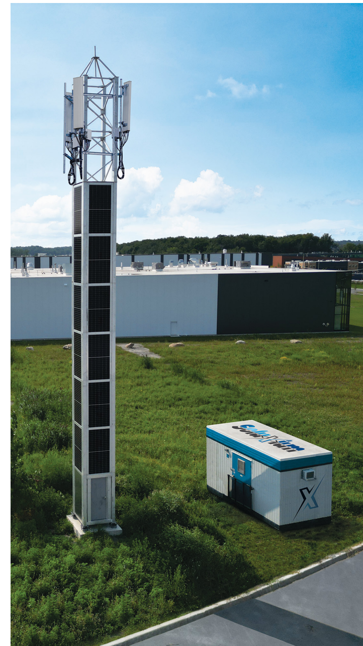
The self-supporting SPT77 in the industrial district of Mascouche.
